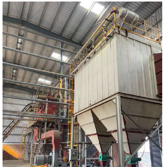
New Biomass Steam Boiler – Capacity : 6 Tons/Hour
