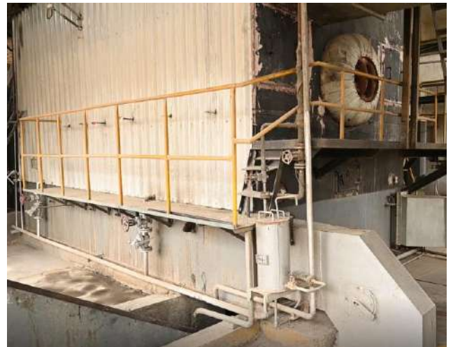
Existing Steam Boiler – Converted from Coal to Biomass
