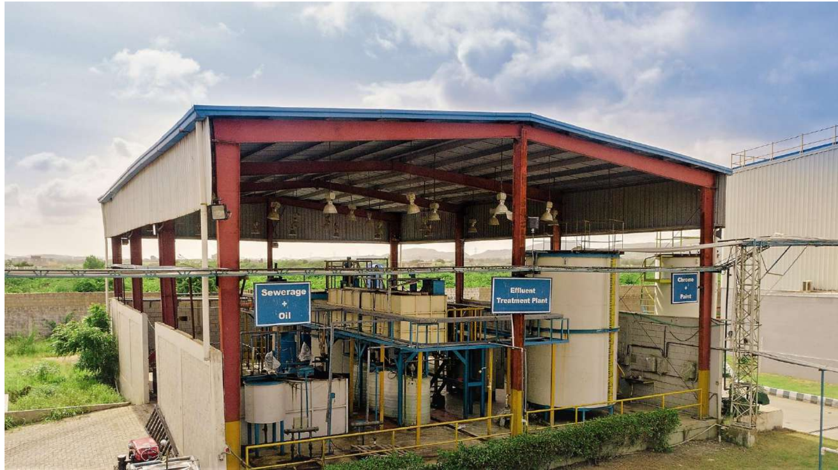
Effluent Treatment Plant
