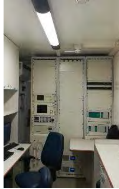
Mud Logging Unit
