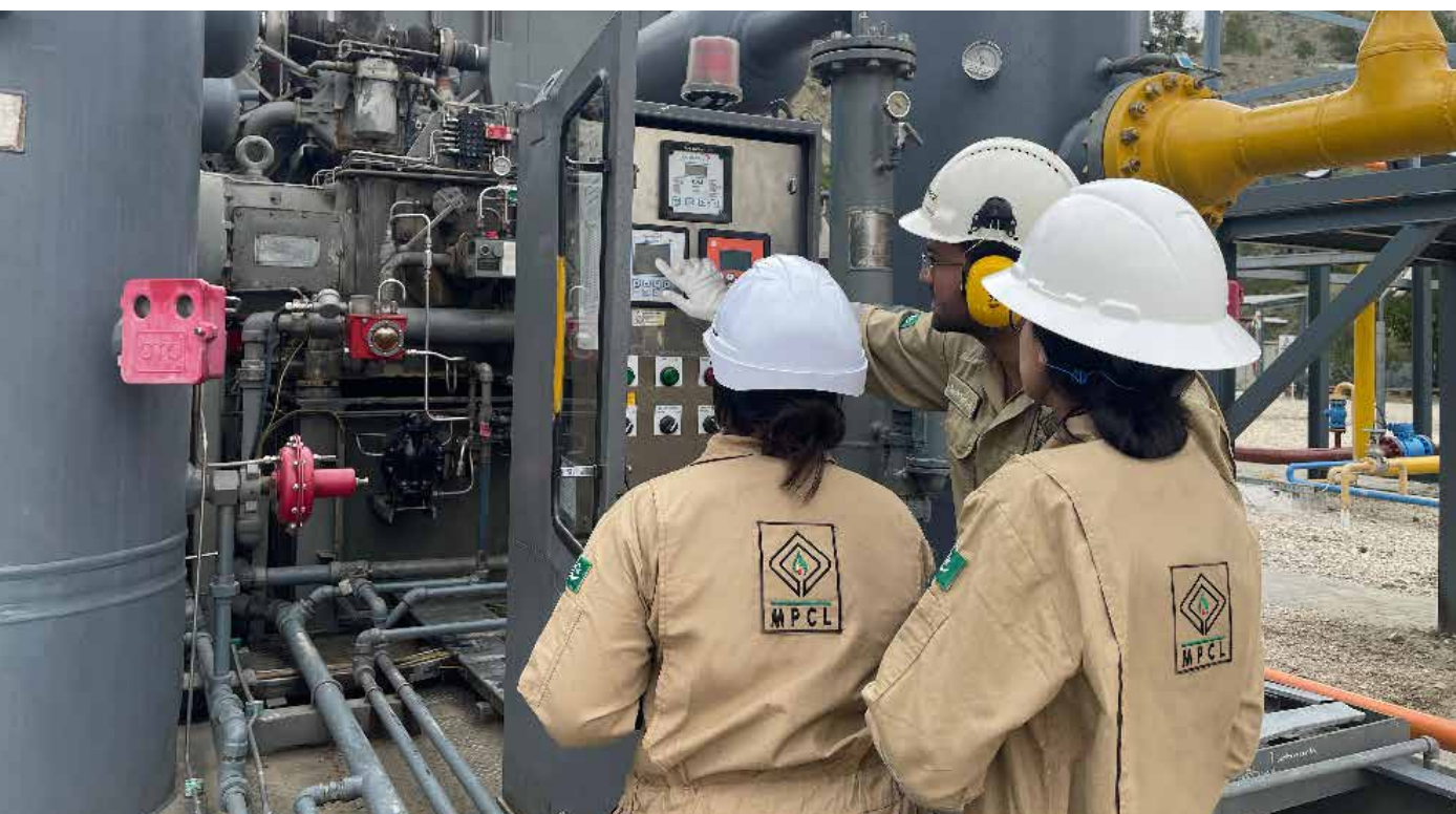
Kalabagh Gas & Condensate Field, Karak Block - KP & Punjab
