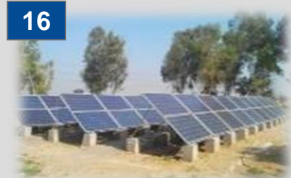
Solar Pumping System
