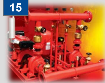
Fire Fighting Unit System
