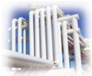
Industrial Gases Pipeline
