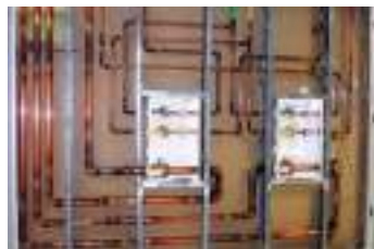
Medical Gas Pipeline
