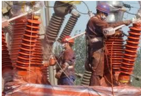
Typical substation insulators being coated
