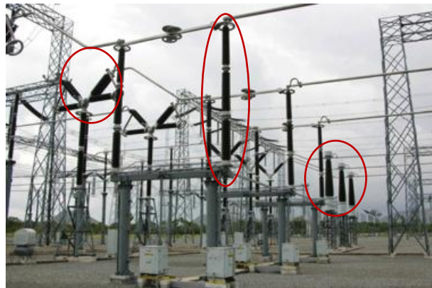
Typical Porcelain Application in Switchgear
