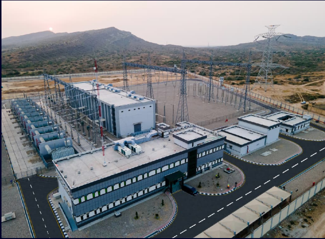
Successful Energization of KKI 500/220kV GIS Grid Station Project
