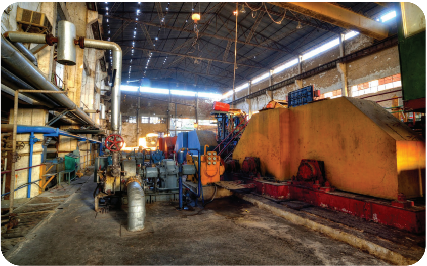
Installed machinery & processing equipment within the production hall supporting sugar manufacturing operations.
