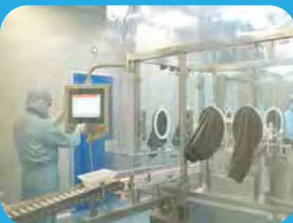
Country's first pharmaceutical facility designed in line with EU and US FDA standards by leading European Pharmaceutical Designers "Telstar Projects"
