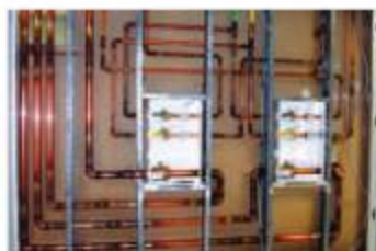
Medical Gas Pipeline
