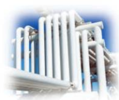
Industrial Gases Pipeline
