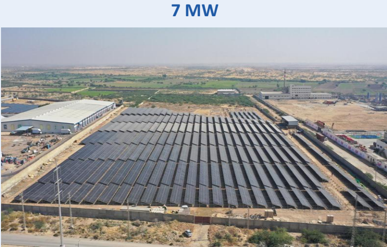
SLM - Solar Park
