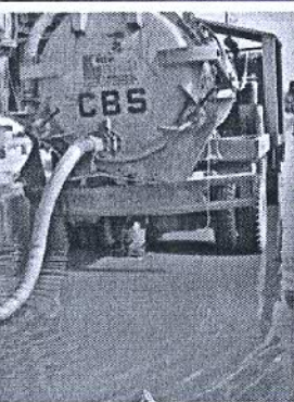
Workers drain stagnant water to ease commuters' movement near canal colony headquarters. REUTERS/AP
