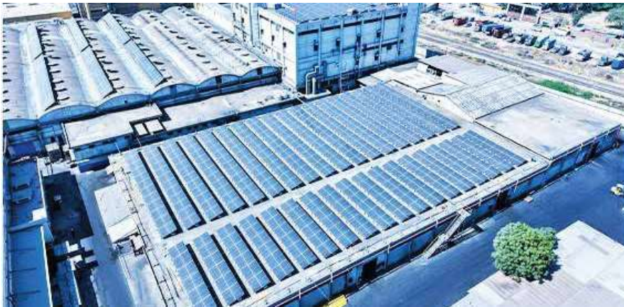
Solar PV at Landhi
