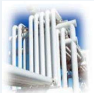
Industrial gas pipelines
