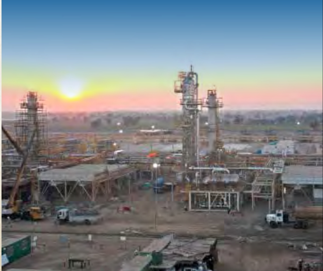
SGPC Plant, Mari Gas Field, Daharki - Sindh
