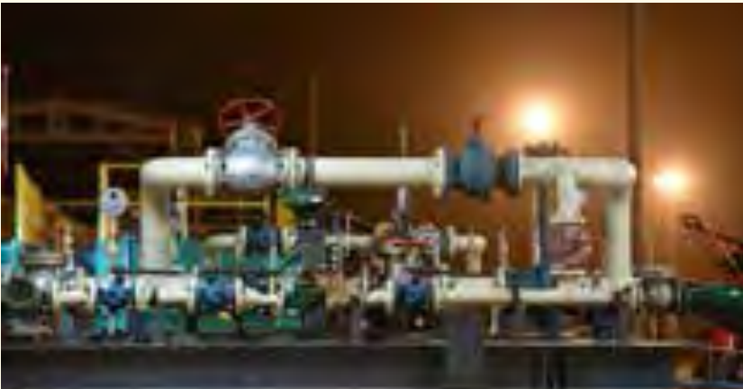
Metering System, Kalabagh Gas & Condensate Field, Punjab
