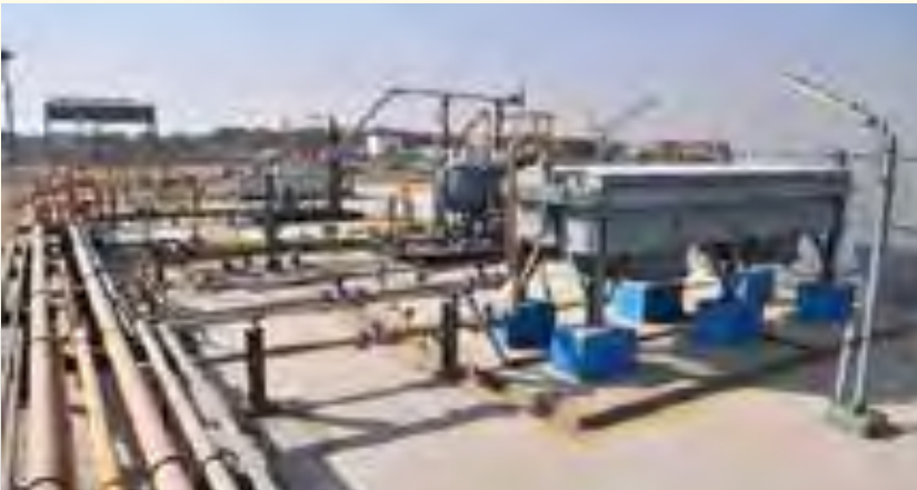
Fin Fan Cooler, Sujawal Gas and Condensate Processing Facility, Sujawal - Sindh
