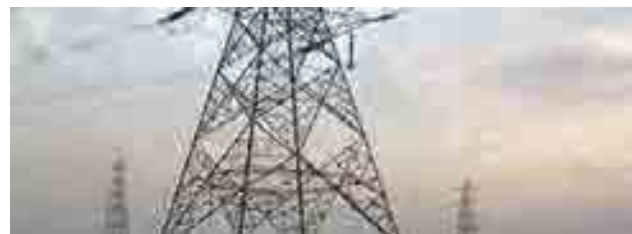
Secure reliable power sourced from CS Energy
