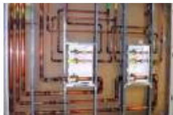
Medical Gas Pipeline
