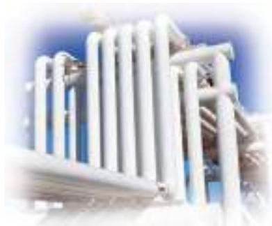
Industrial Gases Pipeline
