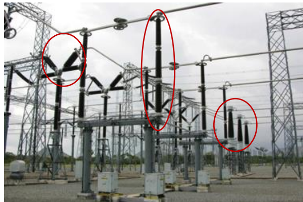
Typical Porcelain Application in Switchgear
