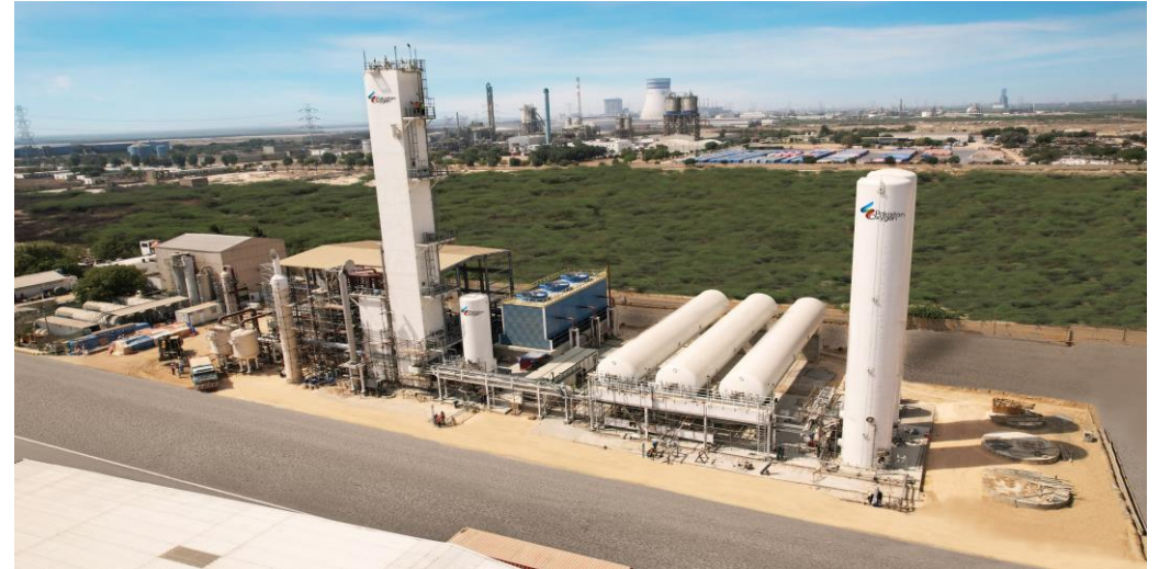
ASU 270 TPD Plant at Port Qasim
