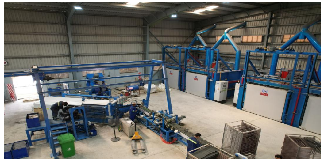
11 TPS Electrode Plant at Port Qasim
